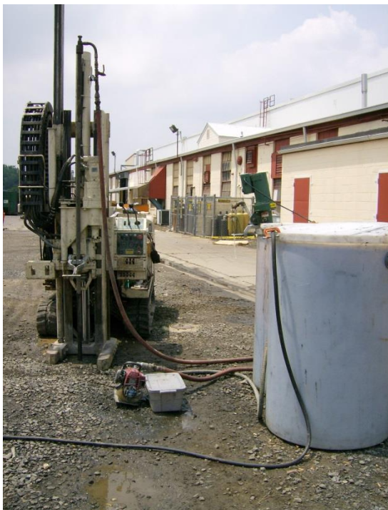
Figure 2: Direct Injection of nZVI in the Field at the Trenton Facility, New Jersey (Photo courtesy of Geosyntec Consultants)
